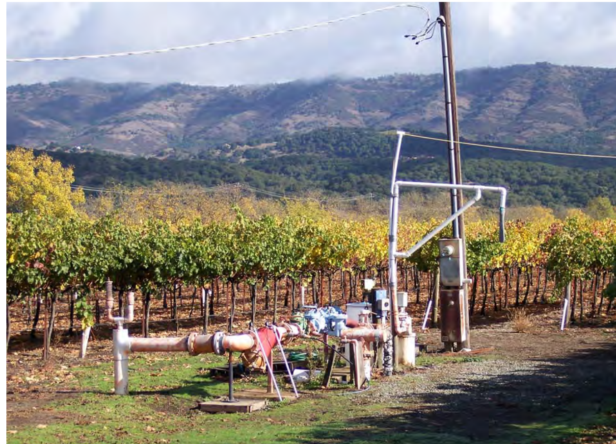
GROUNDWATER WELL, PUMP, AND DISTRIBUTION PIPES
