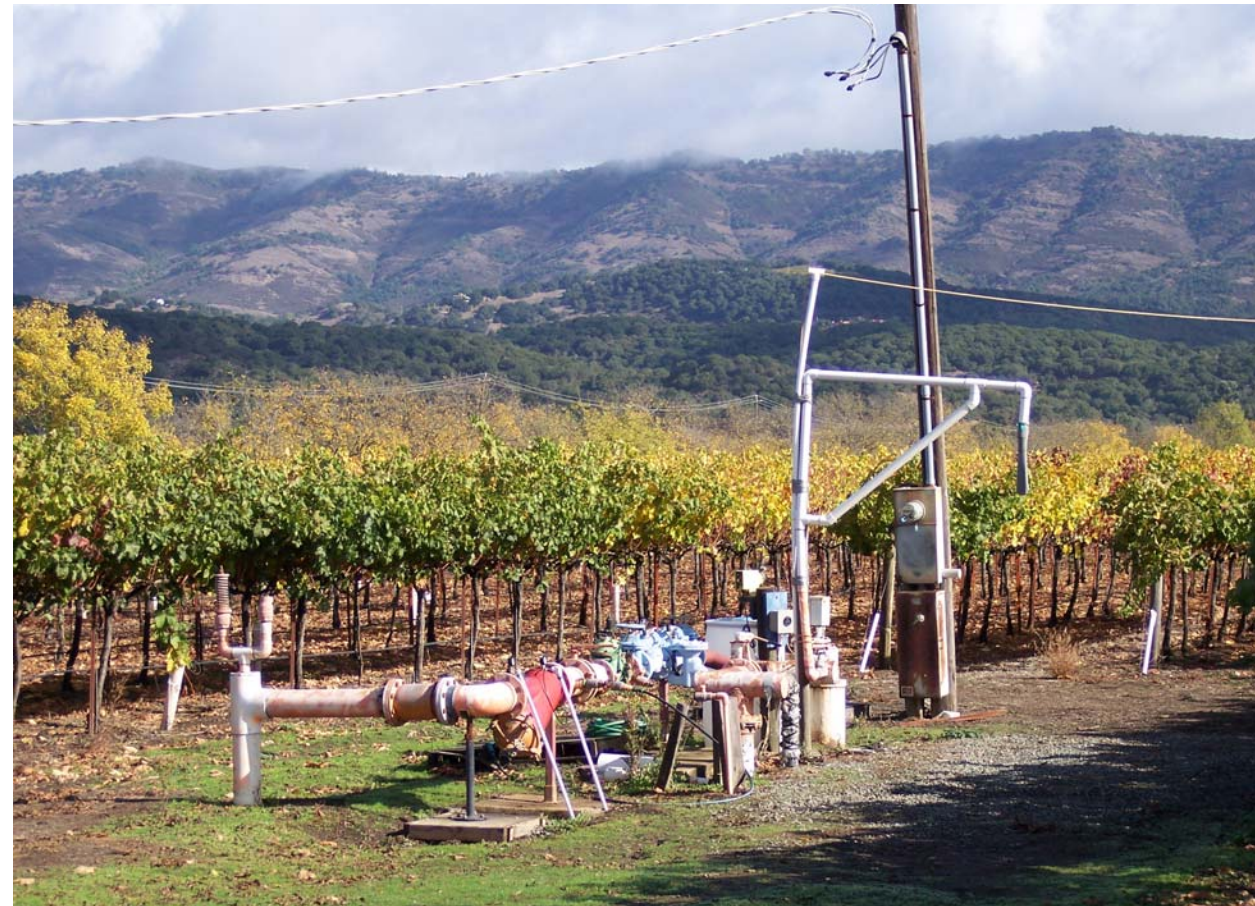
GROUNDWATER WELL, PUMP, AND DISTRIBUTION PIPES
