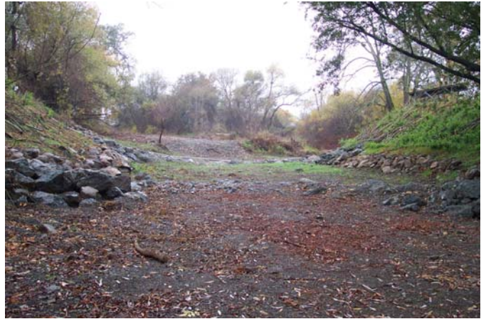
Post-construction: View facing upstream towards remaining gravel bar from 3 rd most downstream weir. (Dec. 2007)
