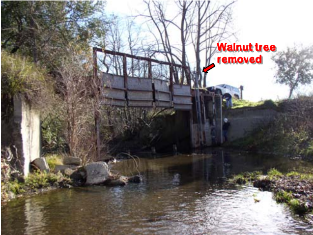
Pre-construction: Looking at the other side of the old seasonal water retention structure. To accommodate the design, a California black walnut was taken down. (July 2007)
