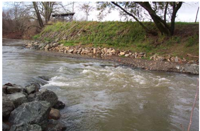
Site observed after flows subsided. No major erosion noted and flows were being directed toward the center of the channel and a pool created. (January 8, 2008)
