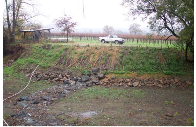
Post-construction: Banks were laid back and stabilized with willow brush mattress and toe rock along the north bank. This boulder weir was installed in place of the sill at a height that is passable for fish passage. (Dec. 2007)
