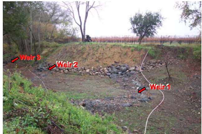
Post-construction: Banks were laid back and stabilized with willow brush mattress and toe rock. Three boulder weirs were installed to allow for easier fish passage and to stabilize the grade of the channel. (Dec. 2007)
