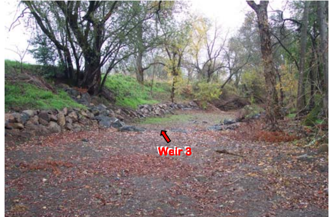
Post-construction: View facing downstream from 2 nd vortex weir towards 3 rd weir. Note construction of willow brush mattress and toe rock along left bank. (Dec. 2007)
