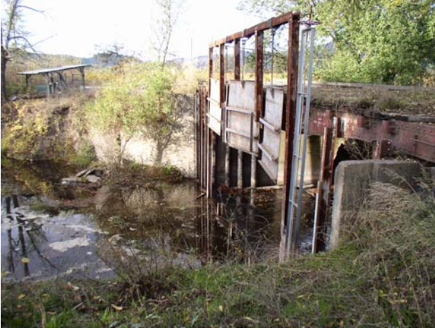
Pre-construction: This old seasonal water retention structure including bridge, wing walls, and sill were removed because it acted as a low-flow barrier to steelhead and Chinook. (July 2007)
