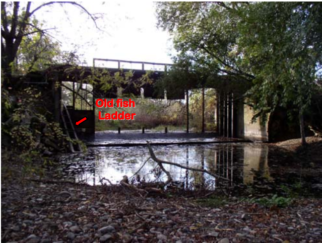
Pre-construction: Facing upstream at barrier, towards concrete sill and apron of the structure which were all removed in addition to the fish ladder on left. (July 2007)
