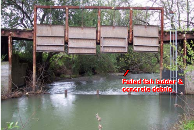
Pre-construction: Facing downstream, towards metal gates. A 2 nd washed out fish ladder and concrete debris downstream of the structure were also removed. (July 2007)
