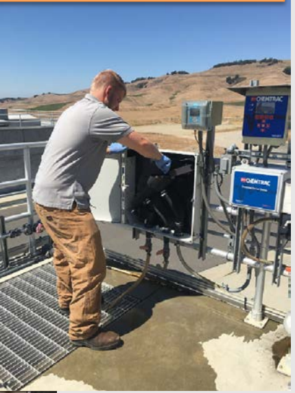
Instrumentation and Controls
