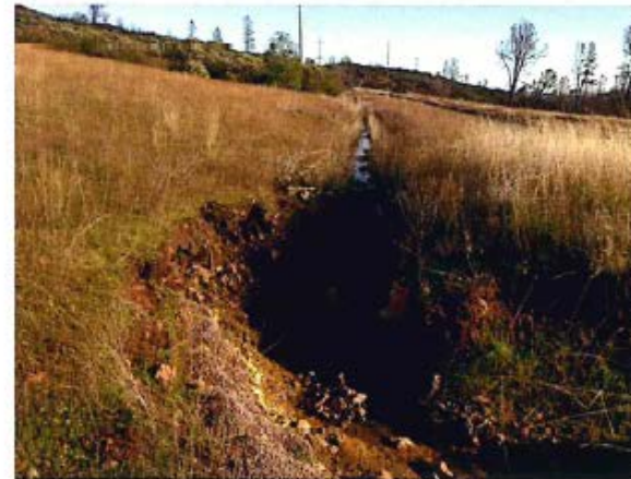
Site 2. The failed ditch has initiated a head cut that threatens serious erosion of this serpentine meadow.
