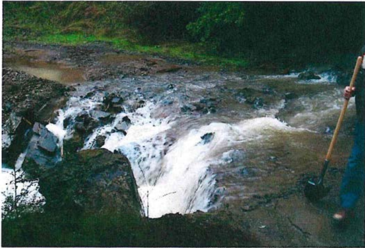
Figure 1. Overloaded and plugged culvert leads to localized flooding and erosion.
