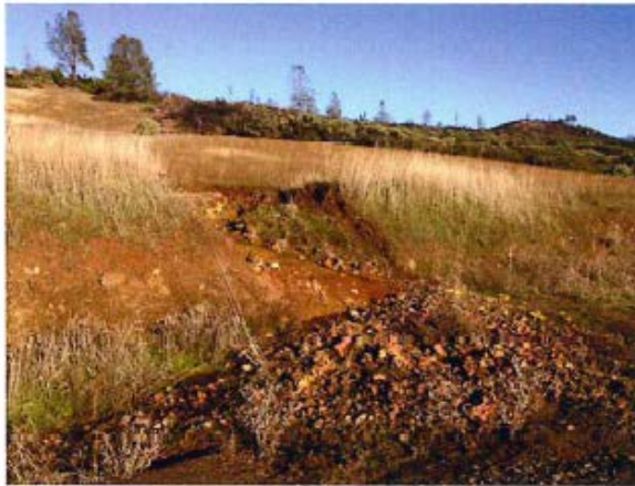
Site 2. A failed drainage ditch from an old pipeline right of way. Similar to site 1, the ditch diverts water from the background sub-watershed into the foreground.
