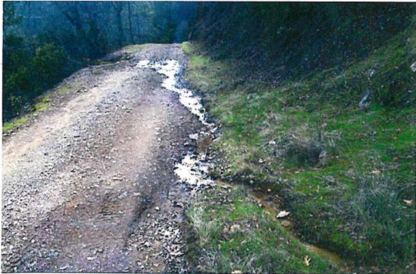
Figure 3. Minor water way from own ditch and erodes roadway.
