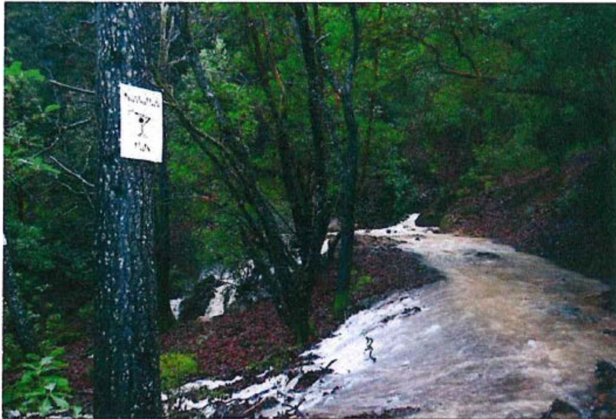
Figure 2. Roadway completely flooded and eroding downslope.
