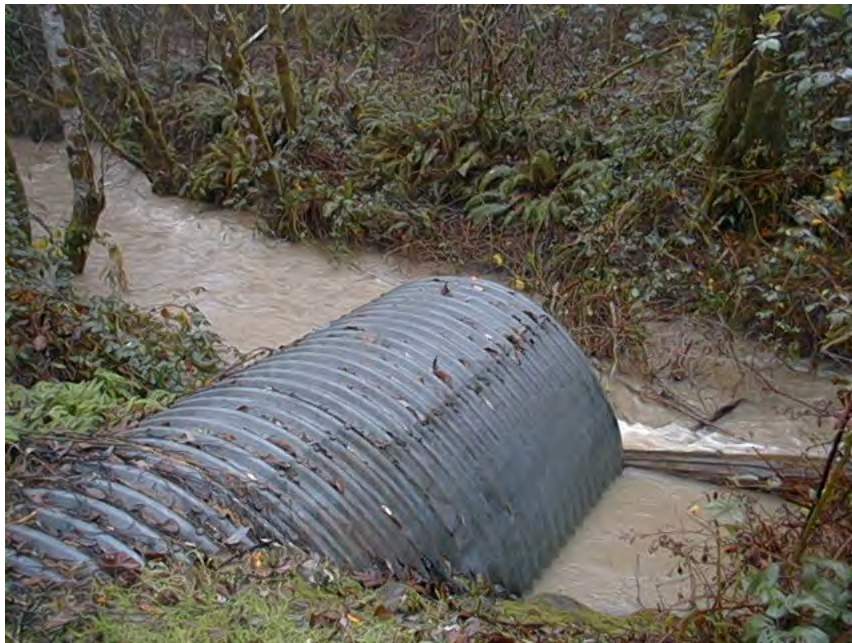
Figure XII-3. Poorly aligned culvert. Note log causing a blockage.
