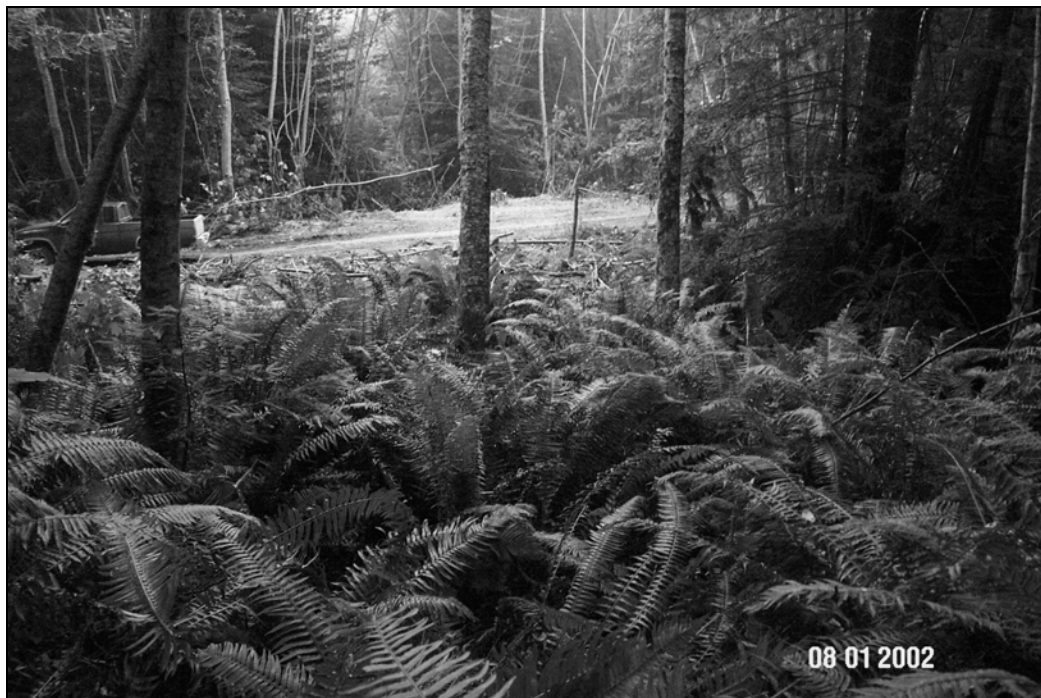
Figure X-D-9. Site # 12, 1300 Road, before excavation. This picture was taken 20 feet above the top of the stream crossing and along the left bank, looking downstream. The stream crossing has been brushed out and is ready to be excavated.
