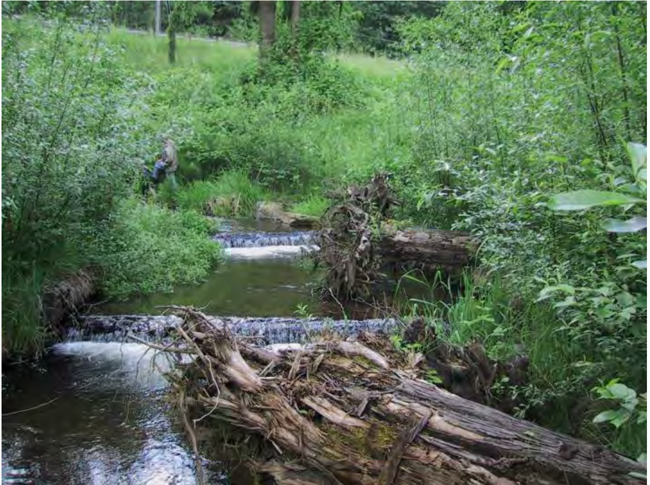
Figure XII-35. Schoolyard Creek bank protection with large wood. No riprap was used on the project. Constructed 2000.
