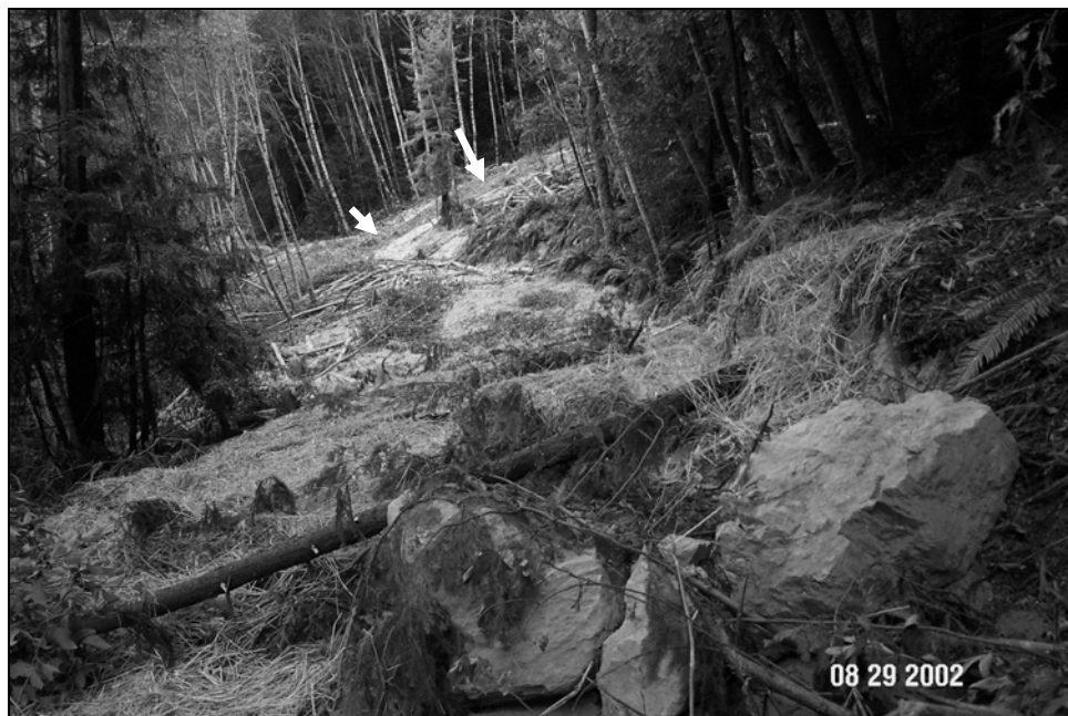
Figure X-D-17. Site #13, 1305 Road, after excavation. This picture was taken from the same viewpoint as Figure X-D-16. The unstable road fill has been completely excavated, mulched and seeded, leaving an outsloped road surface. In the background is one of the main spoil sites for this road. The sloped surface can be seen extending up above the old road bench (see arrows).
