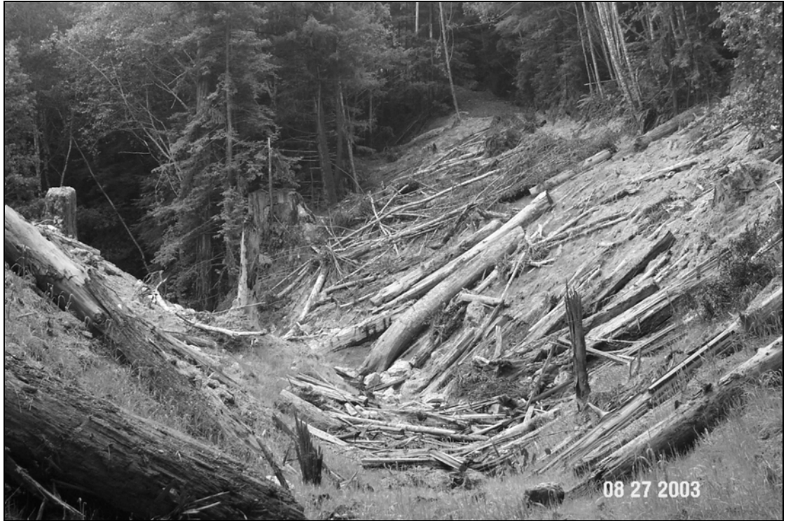
Figure X-D-22. Site #3, 1311 Road, after excavation. This picture was taken from near the Top looking downstream.
