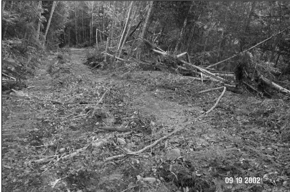
Figure X-D-24. Site # 2, 1312 Lower Road, before excavation. A potential road fill landslide was excavated at this site. Unstable outboard road fill was excavated and stockpiled locally along the cutbank behind the site, creating an out-sloped road surface (see below).
