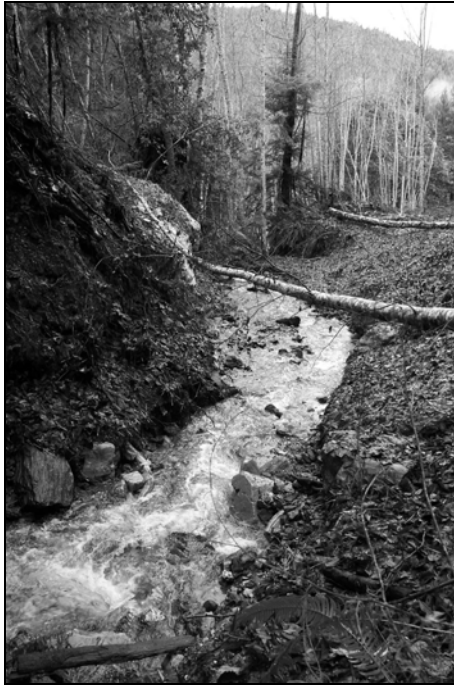
Figure X-D-6. Site # 8, 1300 Road, after excavation. Same viewpoint as Figure X-D-4 during heavy rainfall event.
