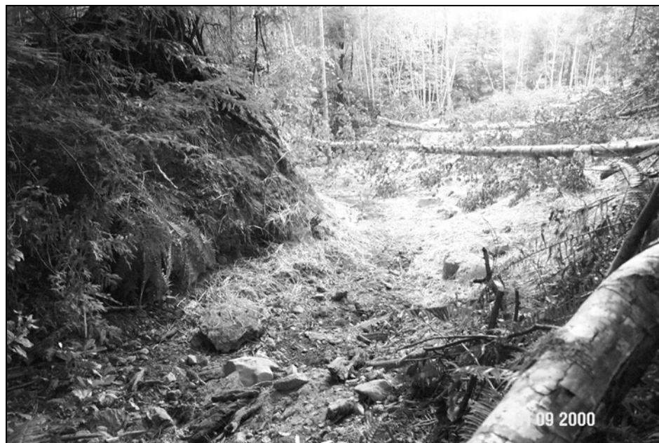
Figure X-D-5. Site #8, 1300 Road, after excavation. This picture was taken from the same viewpoint as above. The stream crossing has been excavated, mulched and seeded. See same view below after heavy rainfall (Figure X-D-6).
