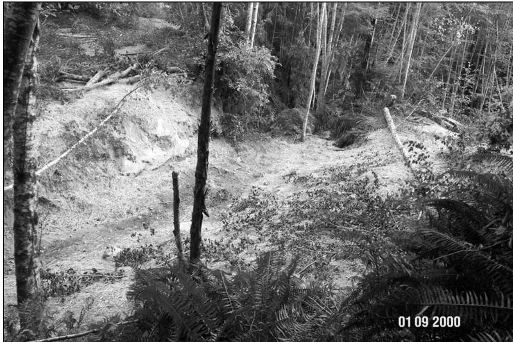
Figure X-D-8. Site # 8, 1300 Road, after excavation. This picture (and Figure X-D-7) was taken 30 feet up the right bank, near the right hinge line of this stream crossing. The stream crossing has been excavated, mulched and seeded. Note location of the two trees for reference.
