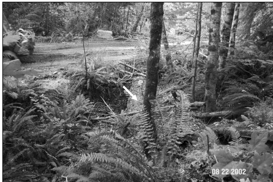
Figure X-D-13. Site # 11, 1305 Road, before excavation. This picture was taken 30 feet above the top of the stream crossing and along the left bank, looking downstream. The stream crossing has been brushed out and is ready to be excavated. A large “Humboldt” log is visible just left of the mossy alder tree in the right-center portion of the picture (see arrow).
